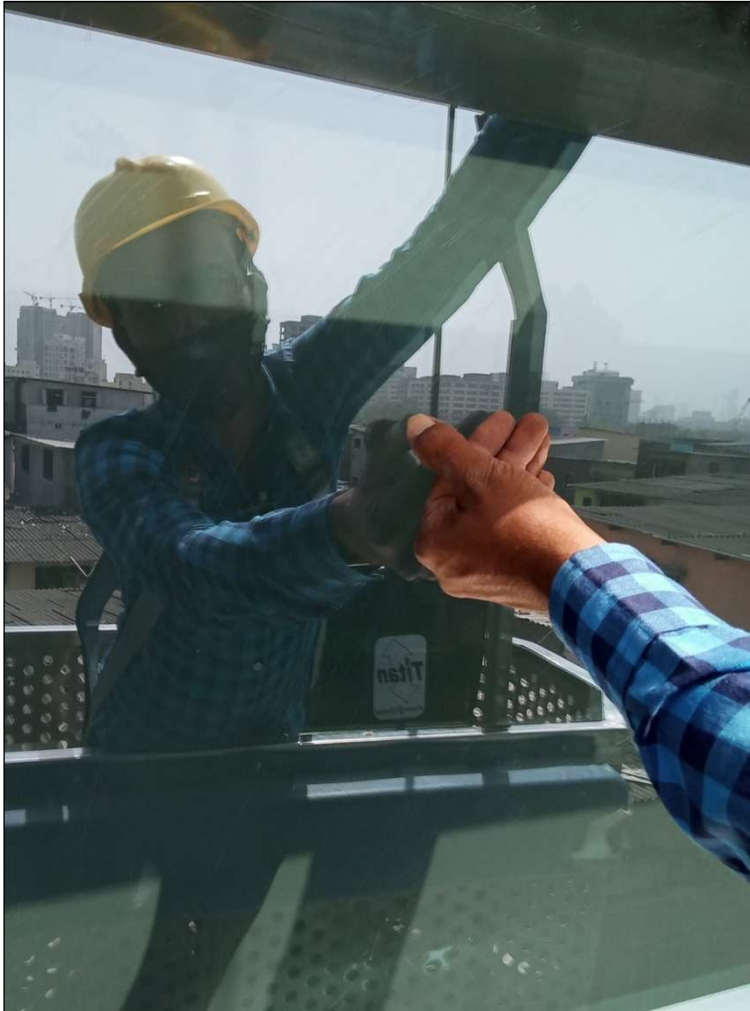
Scratches ( Hairline Cracks) on Glass Floor :3 rd Floor ; Panel below Openable Window
